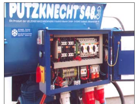
Improved electric control box with automatic motor rotation sense change and safety turn-off
